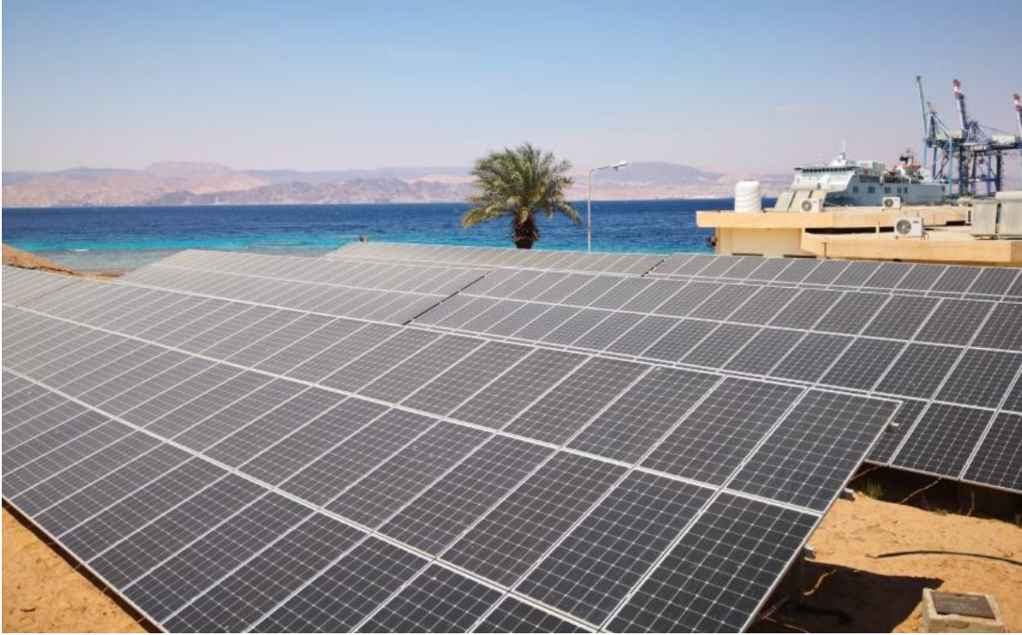
Figure 11 Ground-mounted solar PV system installed at the Marine Science Station.
