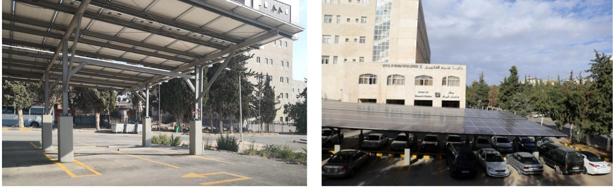
Figure 7 The solar energy project, installed on the rooftops and car parks of the campus.
