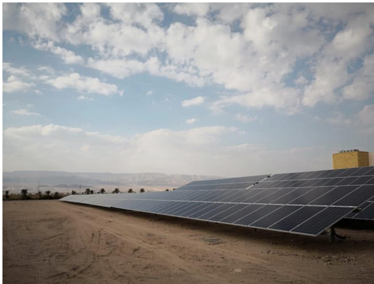
Figure 8 Ground-mounted PV system at Aqaba branch.
