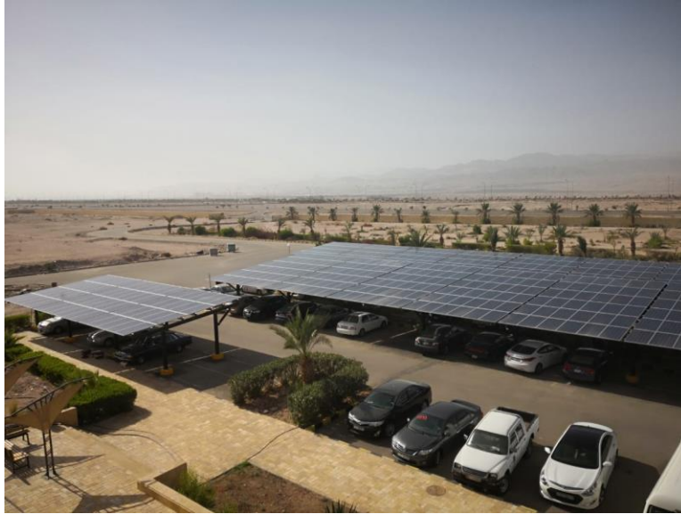
Figure 9 Solar Car park system installed at Aqaba branch.
